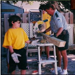
Joshua Bernstein and friend Jonathan Gahagen work on a nature trail for disabled people in Marathon as part of an effort to help Jonathan get his Eagle award. The ranger is Michael Romance, Jonathan's project advisor.
