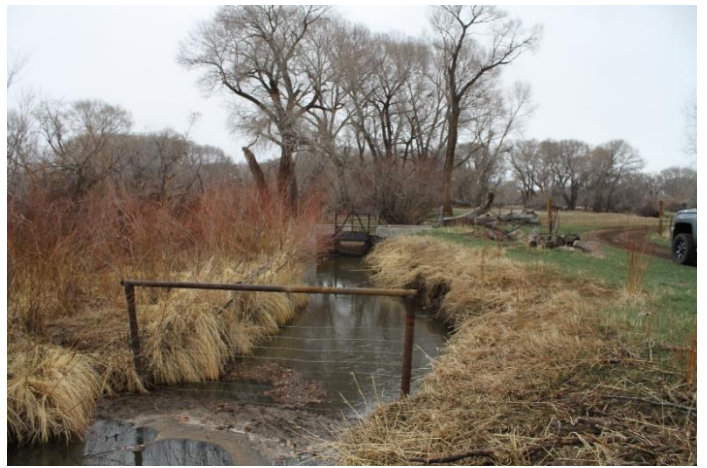
Headgate and trash rack
