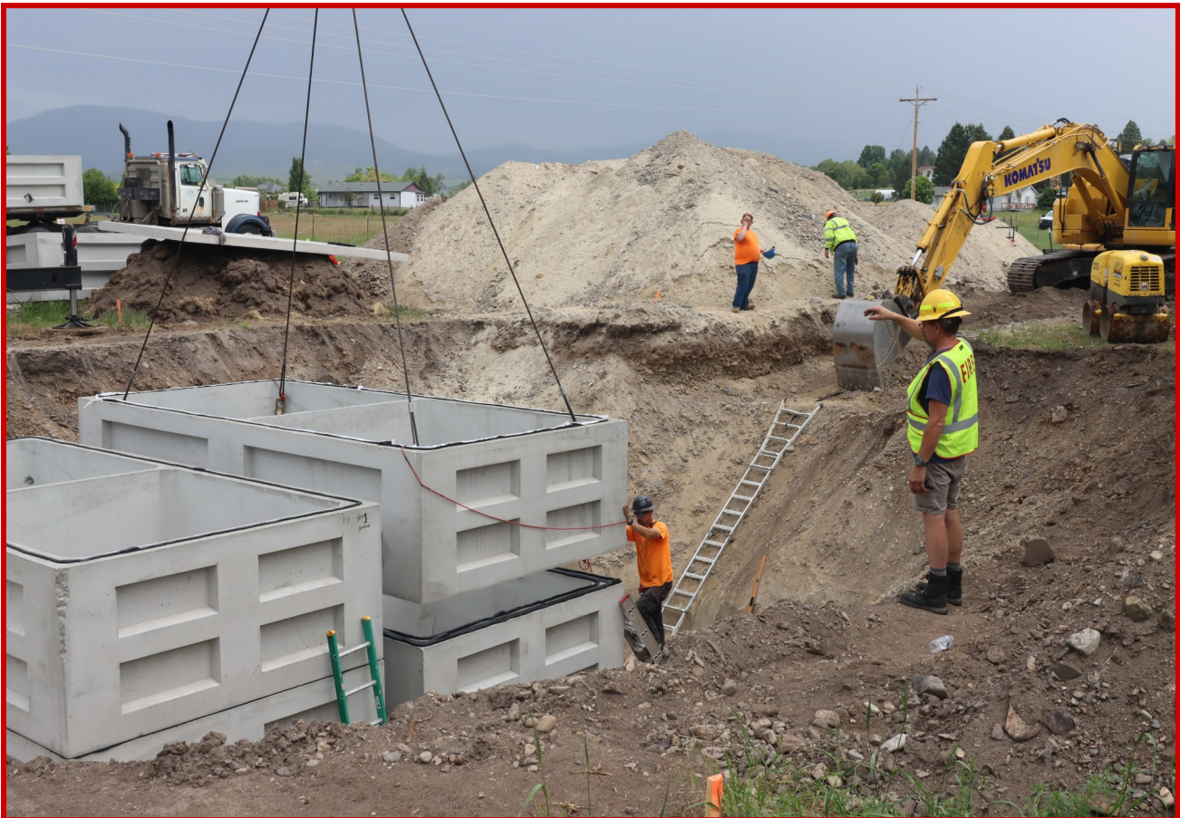
Project Manager Gordon McCullough (in green vest and yellow helmet) directs placement of one of the water tanks for the water fill site.
