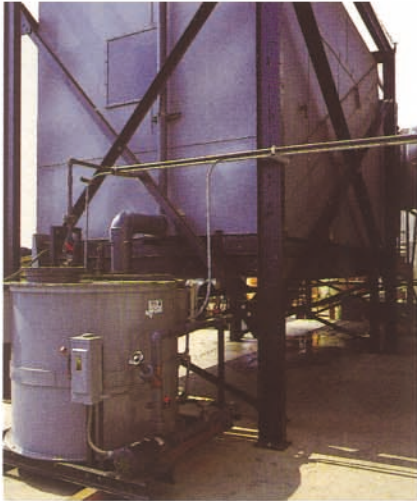
Tri-Mer tank used as scrubber recirculation vessel.
