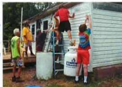
Removing poorly-installed siding
