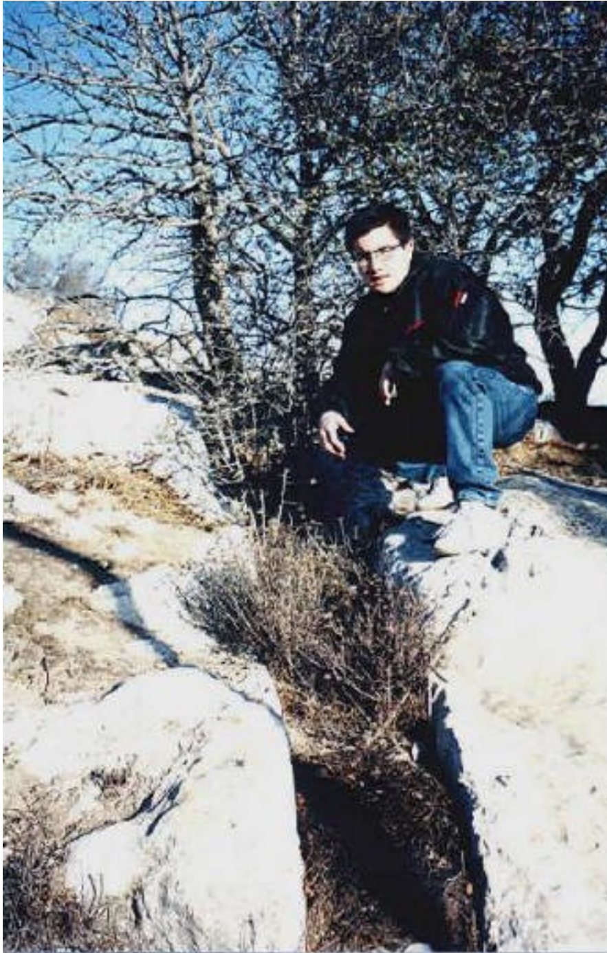
Above: At the top of the escarpment we can see how large the crack really is, but most of the crack has been filled in down near ground level.
