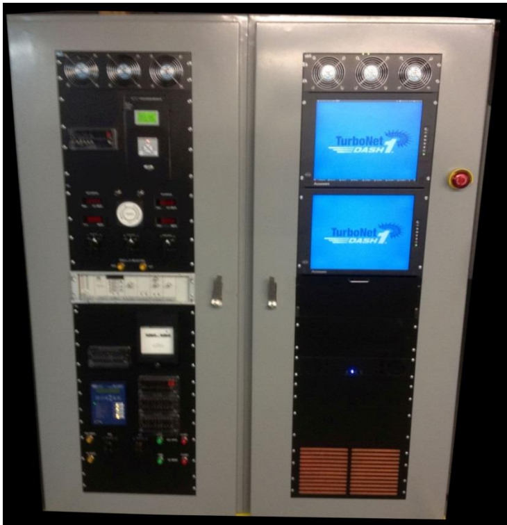
Gas Turbine Generator Front Panel Displays
