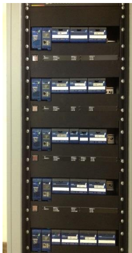
Right Hand Bay I/O Module Door Open Showing Termination Boards
