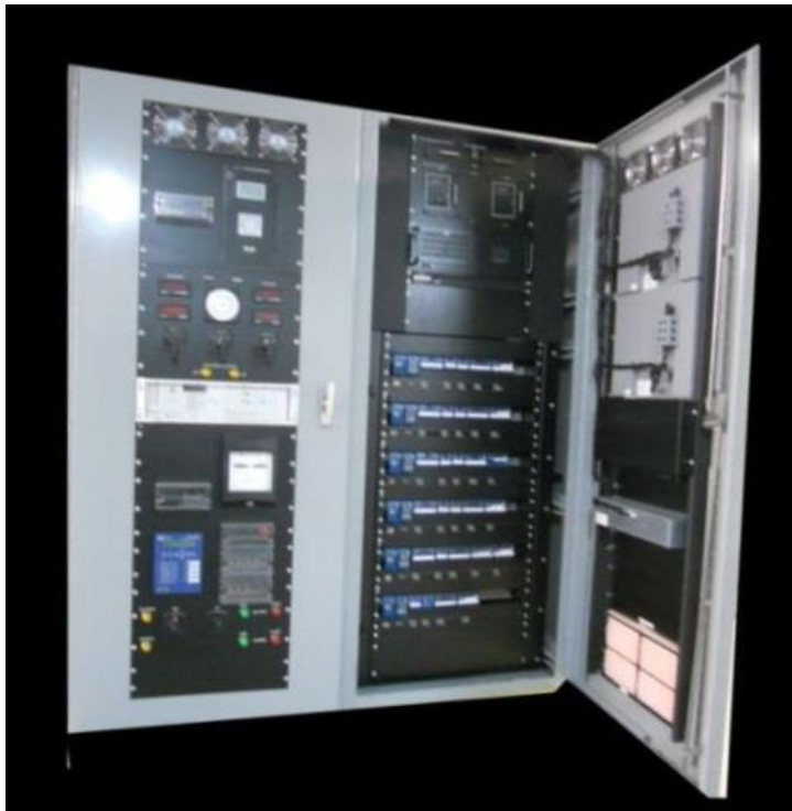
Right Hand Bay Door Open Showing I/O Modules
