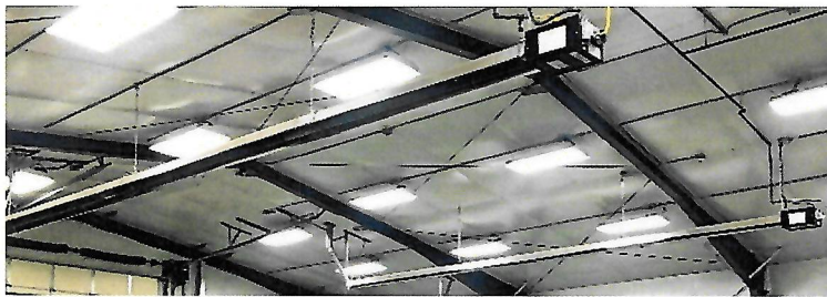
1.5.4 Interior Warehouse Heaters
