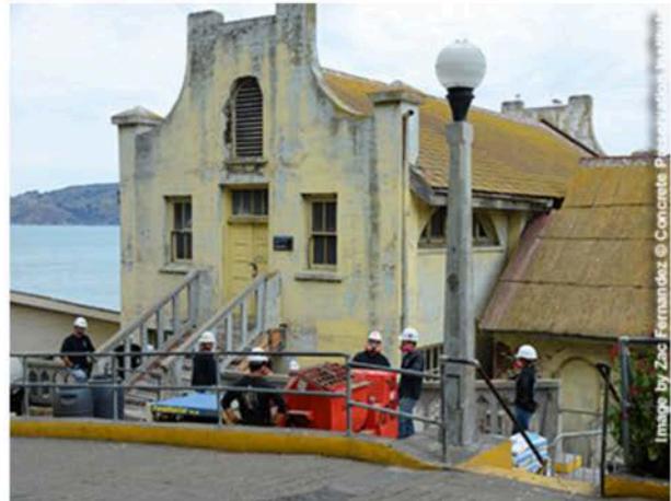
The team prepares structural repairs for a beam, stair stringers, and stairs to the schoolhouse on Alcatraz Island. Image by Zac Fernandez © Concrete Preservation Institute
