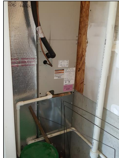
air handler/garage utility room
