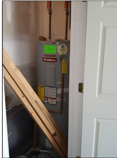
water heater/garage utility room
