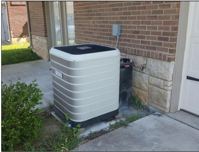
heat pump/rear of home
