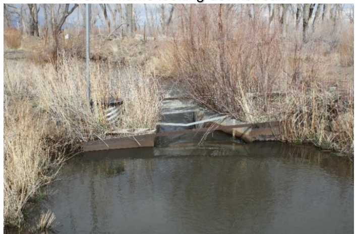
Parshall flume looking downstream
