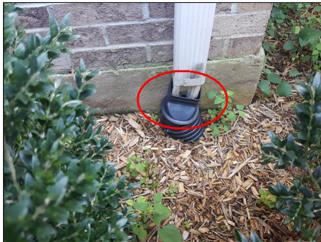
2.3 Item 10(Picture) rear left side of home
