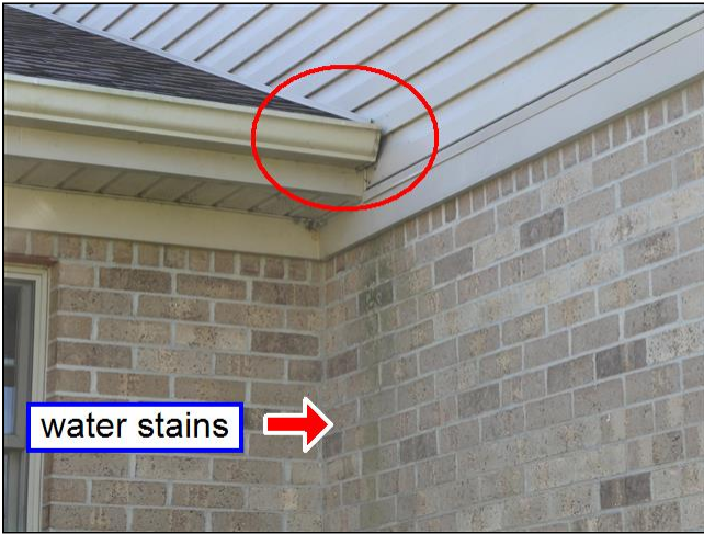
2.1 Item 3(Picture) rear left side of home
