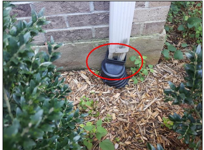
2.3 Item 10(Picture) rear left side of home
