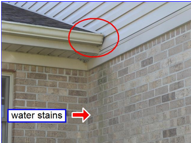
2.1 Item 3(Picture) rear left side of home
