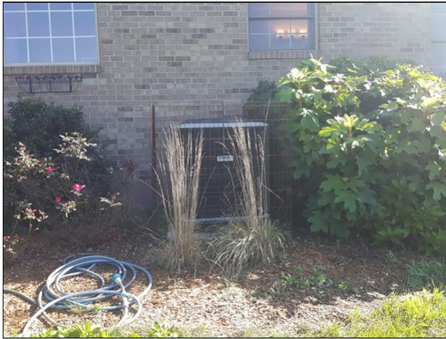
heat pump/rear of home
