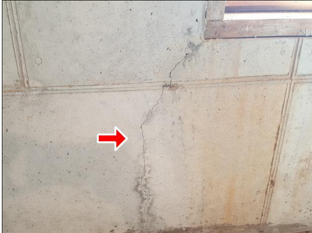
1.1 Item 2(Picture) below basement window
