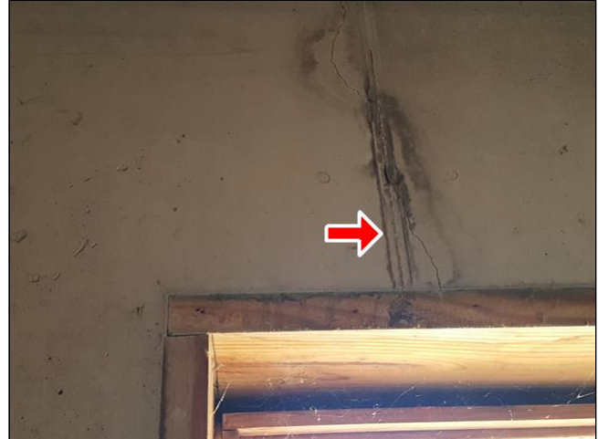
1.1 Item 3(Picture) above basement window
