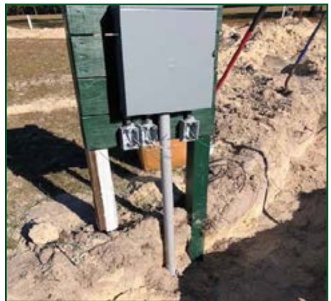
Power hook-up station
