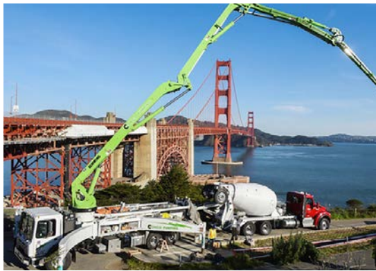
Ready mixed concrete truck and pump setting up just after daybreak at project site
