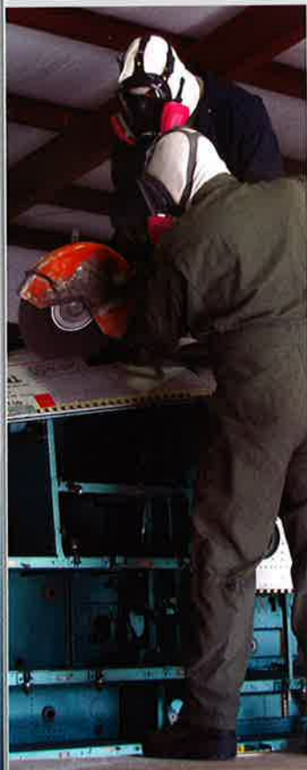
Above: Jim Suzel (SKT/Dayton) and Steve Reeves (SKT/Byron) cut out portions of F-15 structure for inspection. Photo by Channing Duhart
