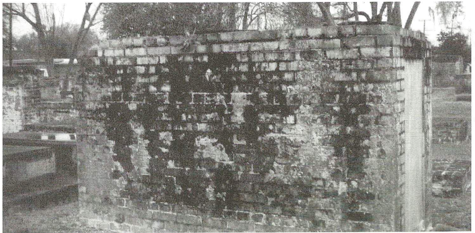
Large brick tomb needing re-stucco and joint repair.
