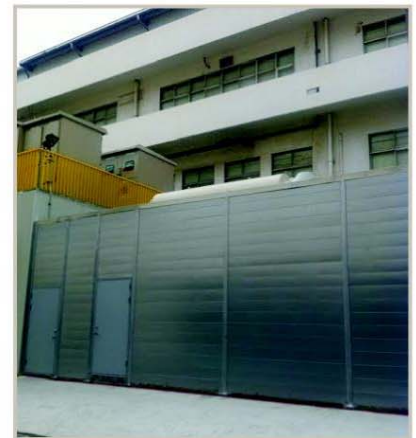
氣體廠隔音牆
