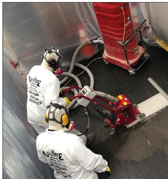
During food processing, hermetically sealed containment in compliance with OSHA standards and upholding GMP/Quality control per client standards.
