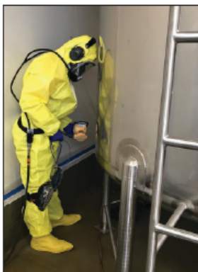
Chemically-resistant secondary containment liner installation performed around tanks filled with chemical compounds. NICI outfitted with continuous-supplied air full-face respirator and PPE to OSHA standards.
