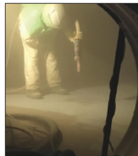
Complete petroleum restoration by OSHA confined space regulations. NICI blasting to satisfy surface preparation requirements in accordance with API standards for 10-year reinstatement.
