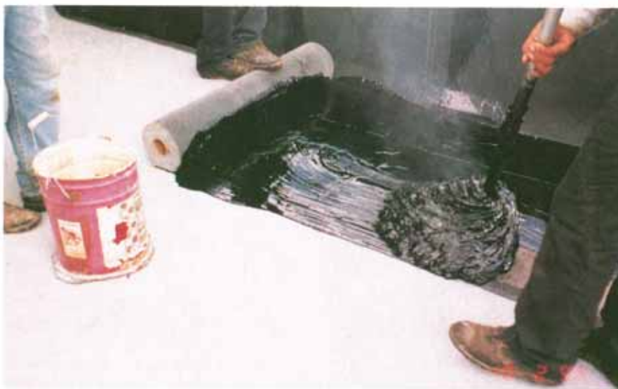
Hot mopping a cap sheet. Cracks from an unprotected asphalt bleed-out.
