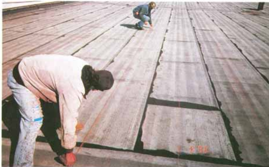
Here contractors chalk lines for the installation of cap sheets - staggering side laps from the base ply.
