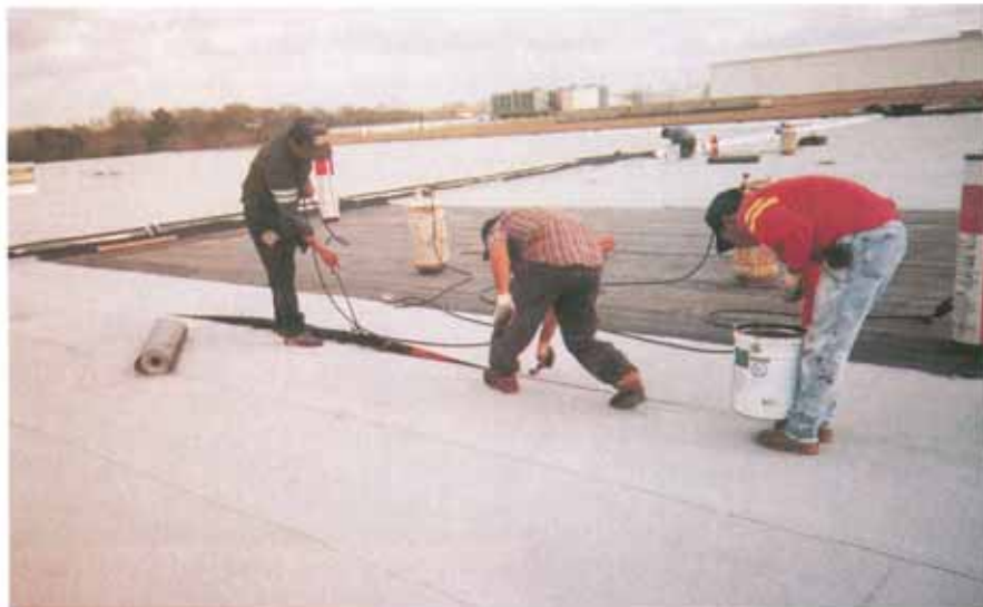
A modified bitumen torch applied cap sheet application – torching side laps, rolling side laps and broadcasting granules in bleed-out.
