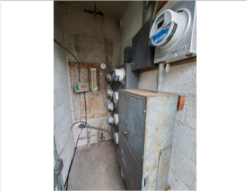
Photo 9 – Village of Dadeland Condominium Association
