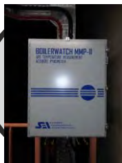
PCU located beside of boiler
