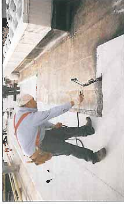
Installer heating granule surfacing at end lap of bottom sheet prior to applying overlying sheet.
