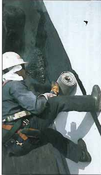
Installer applying downward pressure on cap sheet roll while maintaining roll in close proximity to asphalt mopping source.
