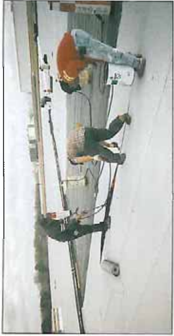
Fusing the side laps of a torch-applied modified bitumen cap sheet utilizing hand-held torching equipment, rolling the heated seam and embedding granules into the bleed-out.
