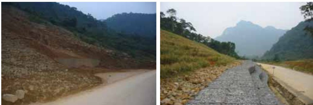
Photo 21: Da Deo Pass, Quang Binh: Left: Vegetation cover is destroyed, revealing ugly and continuous failures of cut slopes; right: Vetiver rows on top of the slope very slowly squeeze down, considerably reducing the failed mass
