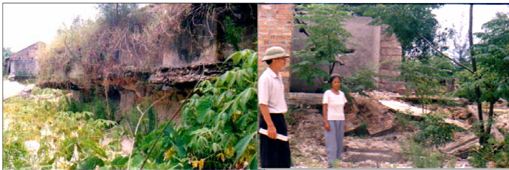
Photo 2: Sand flow in Le Thuy (Quang Binh) in 1999. Left: the foundation of a pumping station; right: this woman's three-room brick house
