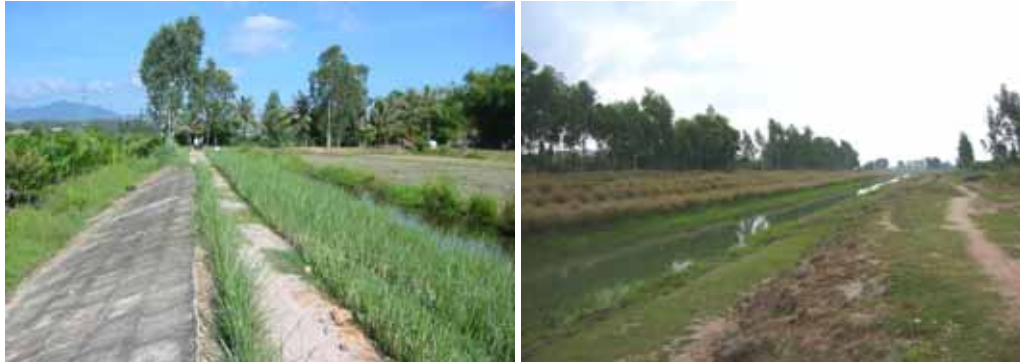
Photo 12: Upstream anti-salinity dike section with traditional concrete riprap facing the river (left) and along a section of the irrigation canal, surface erosion mars the opposite bank (right)
