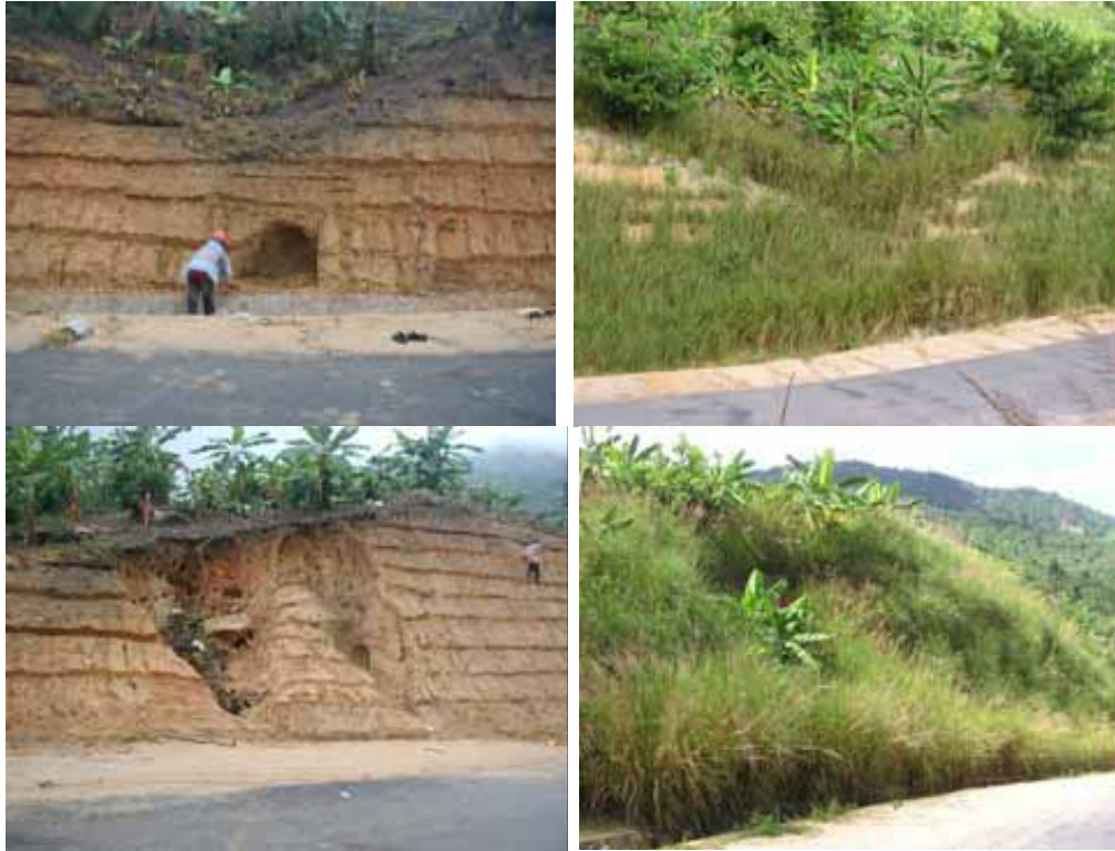
Photo 22: Pham Hong Duc Phuoc, a road protection project in Khanh Hoa province, road to Hon Ba): left two Photos: severe erosion on newly built batter occurs after only a few rains; right two Photos: eight months after Vetiver planting: Vetiver stabilized this slope, totally stopping and preventing further erosion during the next wet season
