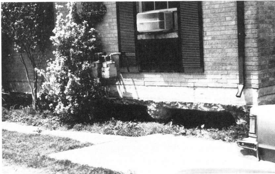
Figure 9-3. Subsidence on organic soils has resulted in structural damage to this house in New Orleans. Source: B. Cox.
