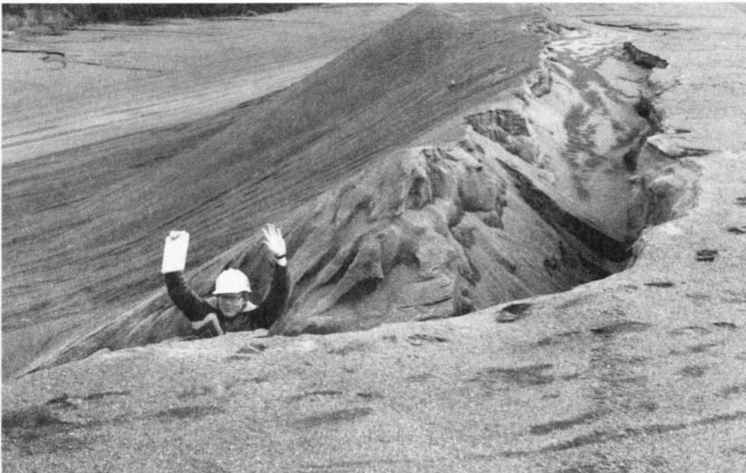
Figure 5-5. Routine dam inspection is a necessary part of a dam safety program. This rather dramatic erosion problem was identified during a routine inspection. Source: Minnesota Dept. of Natural Resources.
