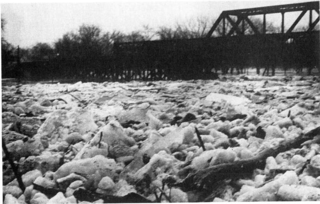
Figure 10-2. This railroad bridge is an example of a man-made structure that can restrict the flow of ice and debris and result in an ice jam. Source: St. Paul District, U.S. Army Corps of Engineers.
