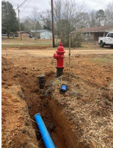
Mize MCWI Water Improvements
