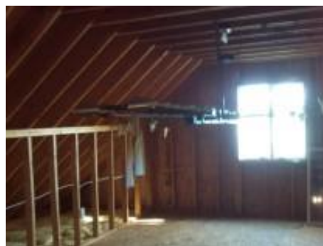
A large FM antenna is mounted in the attic.
