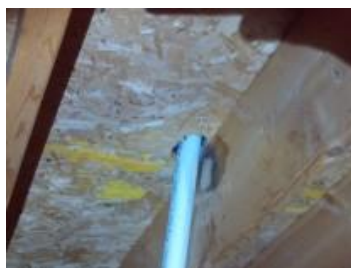
Stains at pipe vent. The moisture meter indicated the area was dry.
