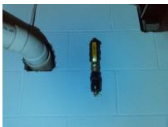
Main water cut-off valve
