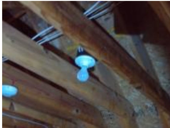
Two attic light bulbs were burnt out.
