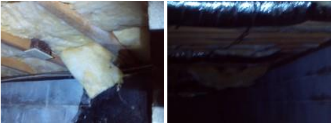
Two pieces of insulation are loose and need to be reattached.
