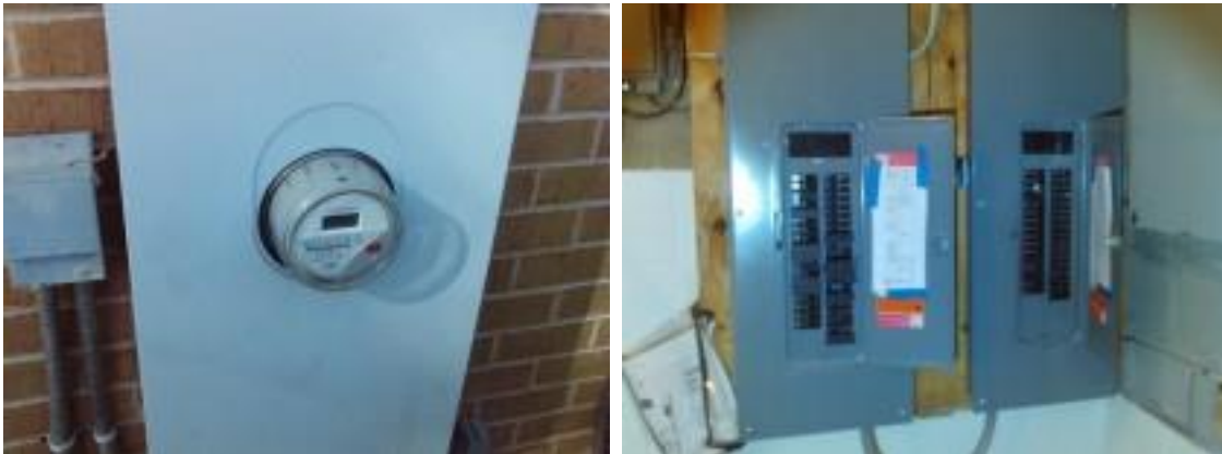
Service entrance and service panel
