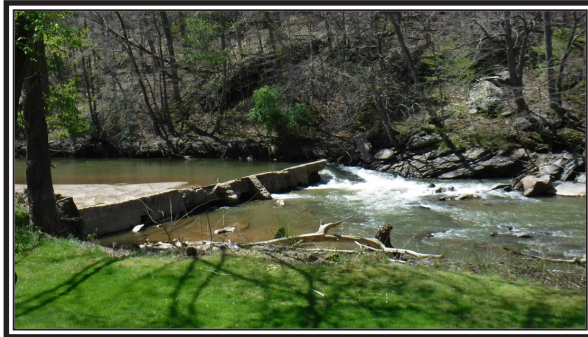
Dam Break from Yard 4/16/2021
