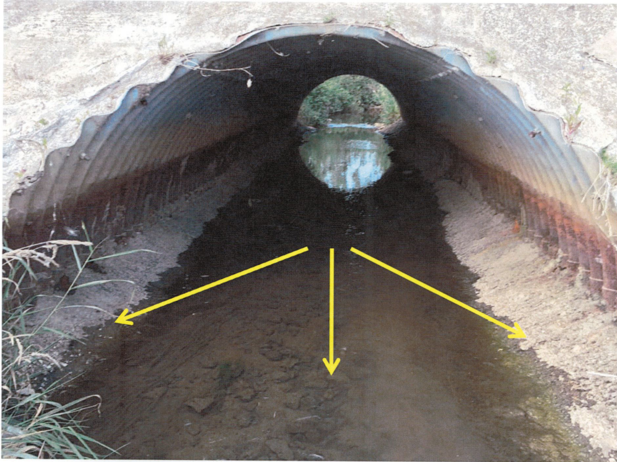
PHOTO 1. Sharp Rd culvert with over 2 feet of concrete and stone base along the bottom, which acts like a dam causing water to backup on Brace Property.
