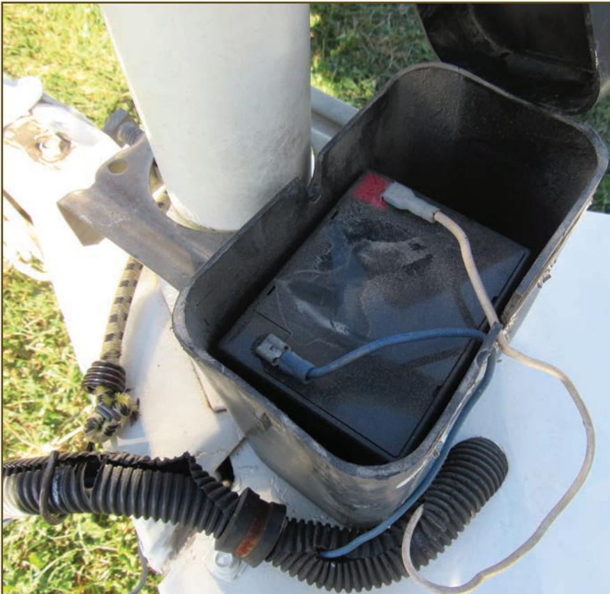
This breakaway brake system's battery is wired to be charged while the tow vehicle is running and is connected to the trailer.
