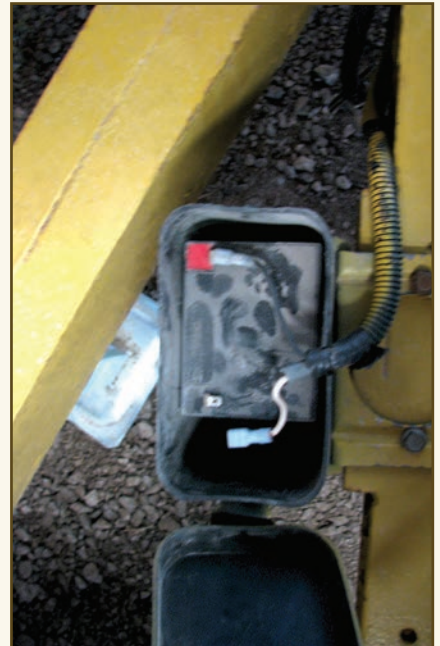
This brake system's battery has loose connections.
