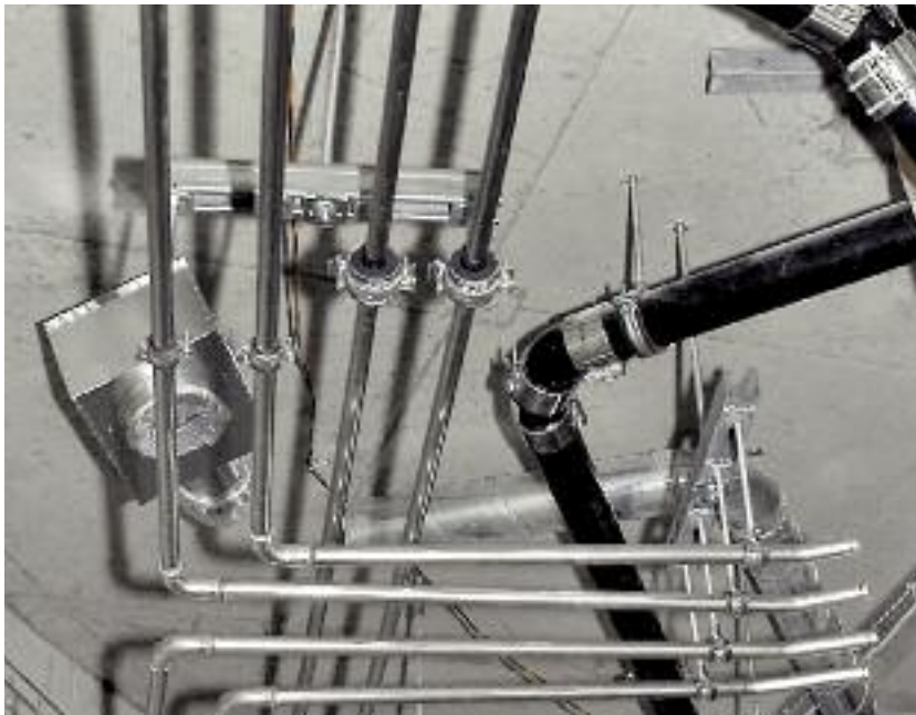
Drinking water, hot and cold water, and heated and chilled water pass through Geberit Mapress pipes, next to Geberit HDPE drainage systems.
