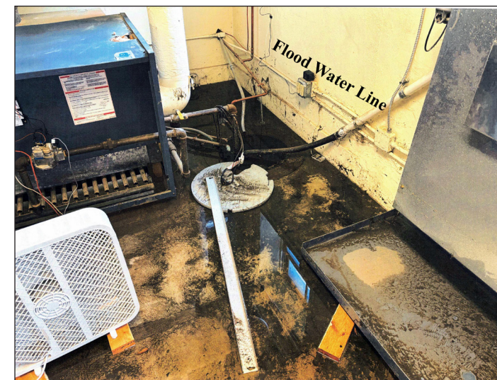
WATER THAT FLOODED THE CARNEGIE BASEMENT really left a mess behind. You can see the water line, showing just how high the water was, which left the boiler inoperable. While the city gave some money to help with the project, the Carnegie still needs $25,000.
