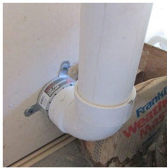
Elbow joint from the basement ceiling joist into the garage. Note the fire stop collar.
