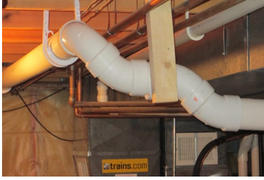
The PVC elbow configuration allows the exhaust pipe to go under the heat ducts and water pipes.
