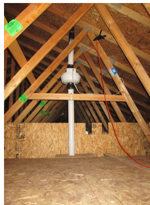
New 192 square foot of storage space and installed exhaust fan. The switch can be used to turn off the fan.
