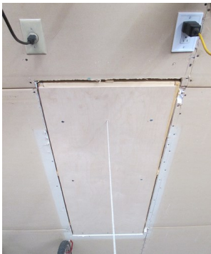
The attic ladder in the closed position - still needs the 5/8 drywall fire barrier to get the garage ceiling up to code
