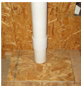
The small piece of OSB was cut to fit and placed before the connecting collar and pipe about the collar was installed.
