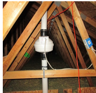
Exhaust fan and electrical switch with an added 2 x 4 cross brace.
