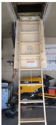
Fully opened ladder - note the signatures of the people who assisted with the installation.
