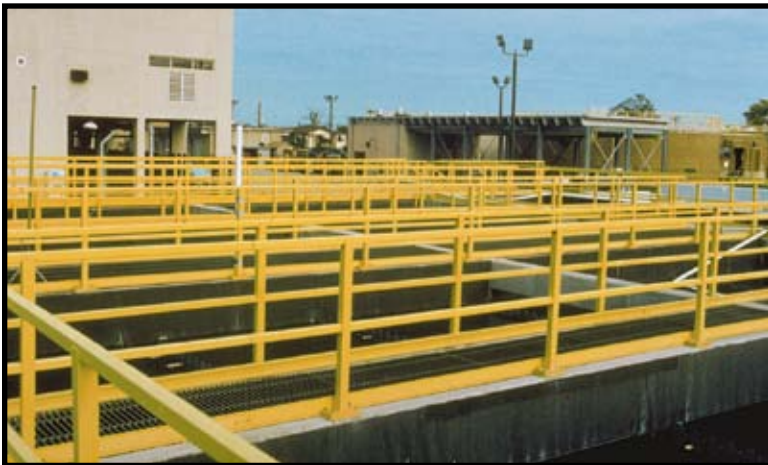
Square tube handrail manufactured with Dynaform component products offer long life in the corrosive environment of this wastewater treatment plant.
