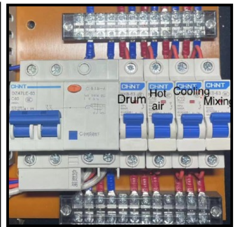
NEW CIRCUIT BREAKER SYSTEM
