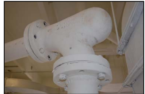
This HammerLoy Series Smart Elbow from HammerTek, Landisville, Pa., is one of 14 such elbows installed at the Upper Occoquan Water Reclamation Plant in Centreville, Va. to eliminate pipe failures in the conveying line. After more than four years in operation, all of the Smart Elbows continue to perform as specified without a single pipe failure.
