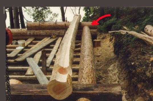
Window Log In Place (red arrow) With Next Log Ready For Borate and Fiberglass Insulation
