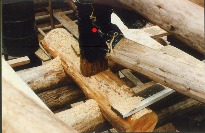
Middle East Support For West Ridge Pole: Setting On Crossbeam Placed Between The Two Central Walls West End Of Northeast Purlin Is Attached To Support
