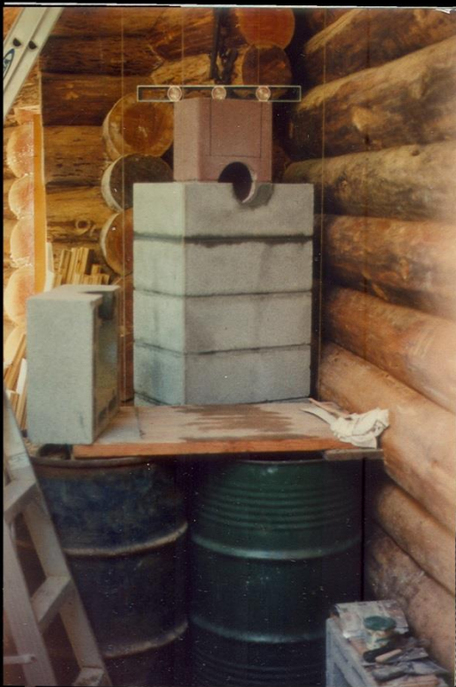
Bottom Of First Pipe Hole Cemented Checking Level Of Pumice Liner Top Half Of Hole To The Left
