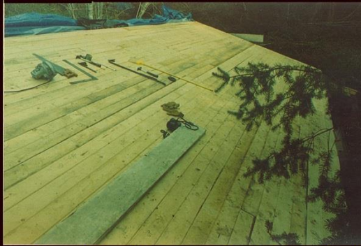
Southeast Roof Looking East This Part Is The Largest Expanse @ 36 feet by 14' 6"
