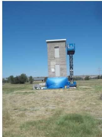
Working on the Memory Tower. The Memory Bricks are protected by the blue plastic, August 2020
