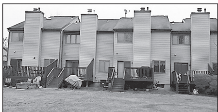
The project included removing original wood clapboard, structural repair and the installation of vinyl siding.
