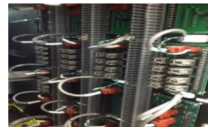
Left Hand Bay Termination Boards
