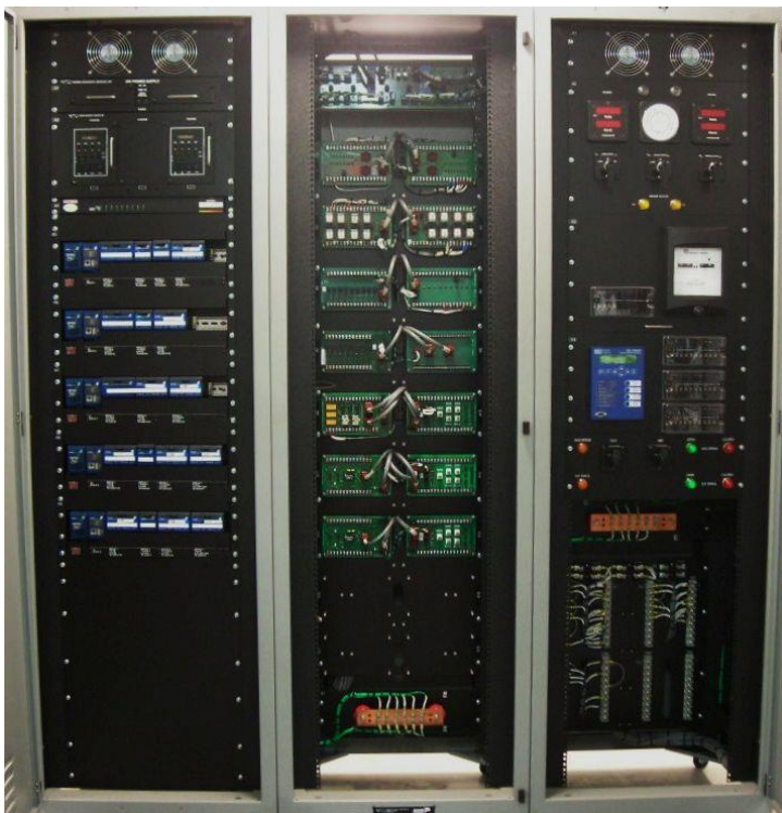
Steam Turbine Generator Cabinet with Auto Sync (Bay Doors Open)
