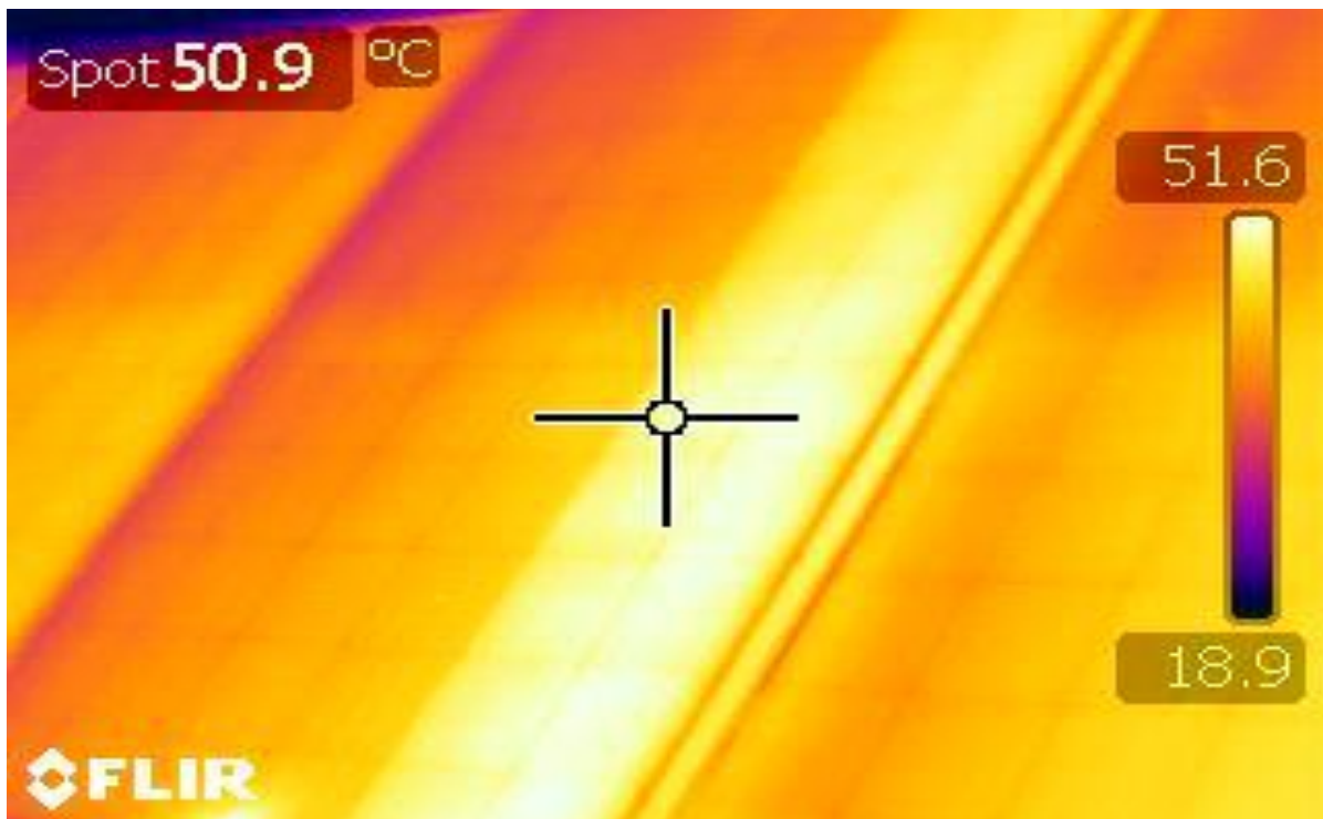
Fig 8: Bypass diode problem module
