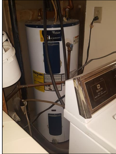
2nd water heater/basement washer dryer room
