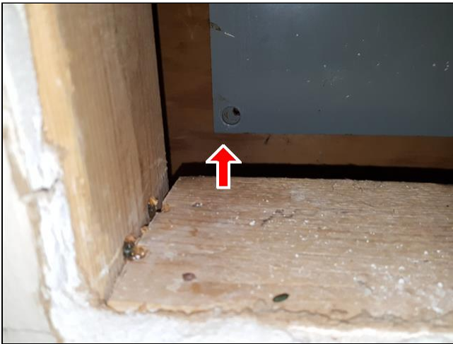
9.2 Item 1(Picture) main panel
