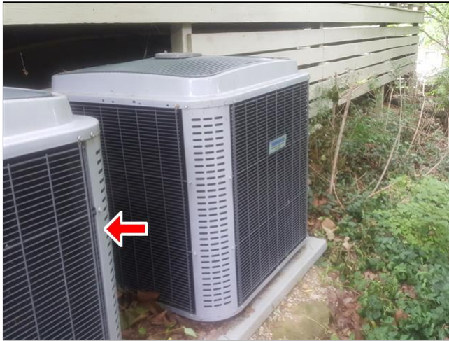
heat pump/right side of home
