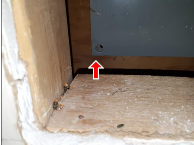
9.2 Item 1(Picture) main panel
