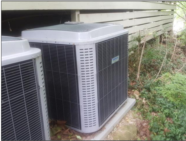
heat pump/right side of home
