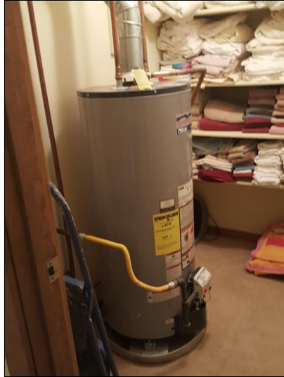
water heater/upstairs closet
