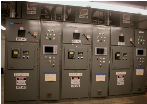
Award winning: Lake Lanier Raw Water Pump Station Lake Lanier, GA
