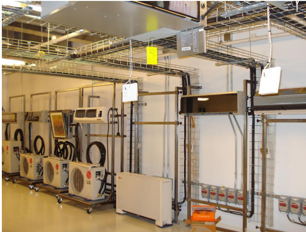
LG Air Conditioning Academy Training Laboratory, Alpharetta, GA
