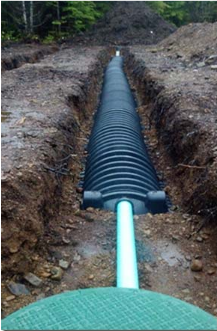
This is a conventional gravity system with chambered trenches. The green lid you can see at the bottom of the picture is the access to the d-box.
