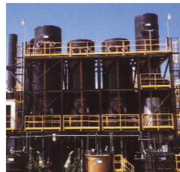
Tri-NO x Multi-Chem vertical system applied to nitrating oven.
