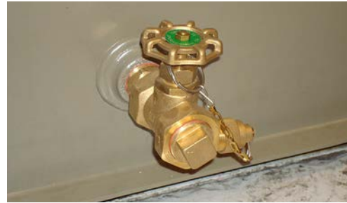
Figure 3. Drain valve with sampler
