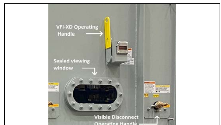
Figure 8. VFI-XD transformer with visible break
