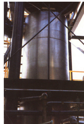
Quencher system under multi-stage gas scrubber
