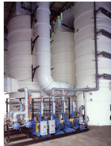
A 28,000 CFM Cloud Chamber scrubber
