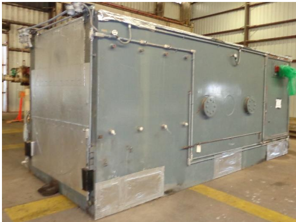
STEAM TURBINE AND GENERATOR ENCLOSURE (LEFT VIEW)
