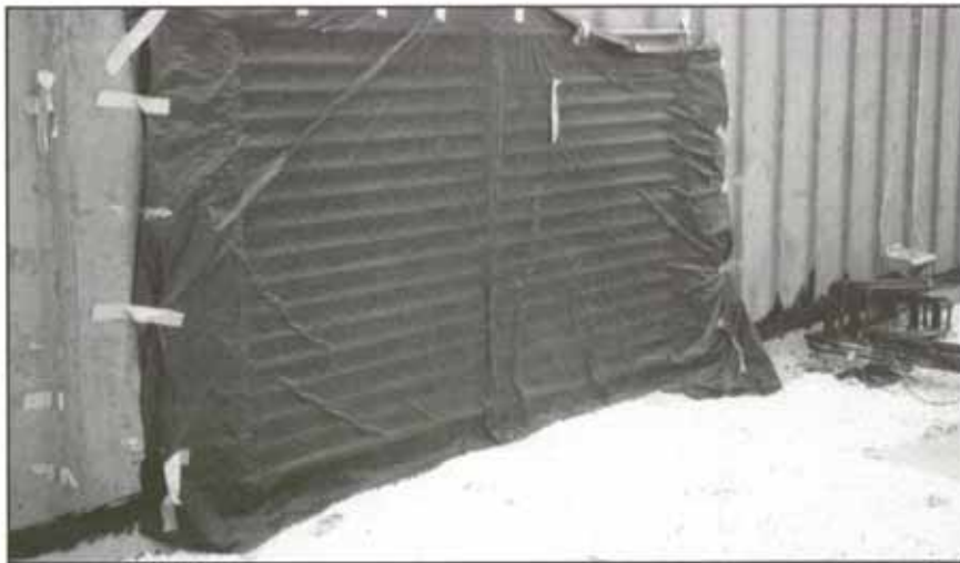
Lower intake in wall covered with plastic sheeting to prevent fume infiltration.
