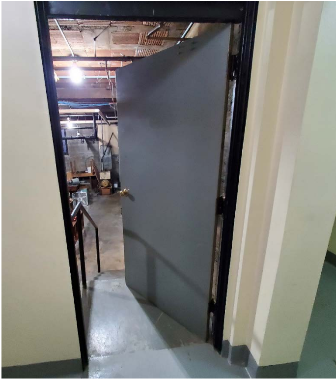
Door 4 Interior Mechanical Room
