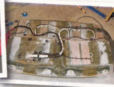
12. The 12-volt power wires were mounted on the backside of the console to keep the music-carrying cables on the front side free from interference.
