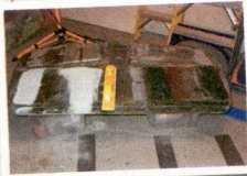
9. Aluminum plates were "bedded" onto the backside of the structure using Evercoat's Tiger Hair fiberglass reinforced filler.
