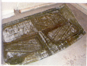
5. View of the mounting surfaces of the composite structure prior to the application of fillers.
